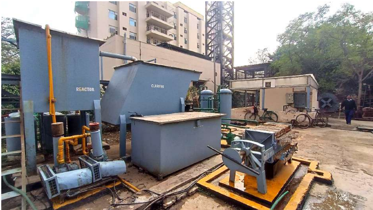
Photograph :- 350 KLD STP & 25 KLD ETP Area
